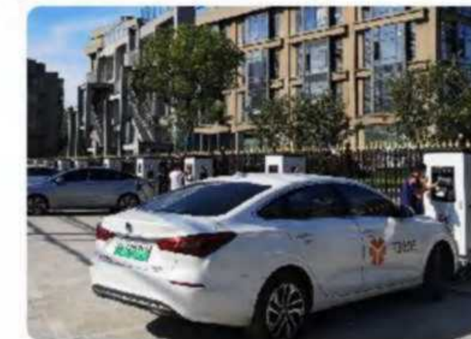
Community charging station
