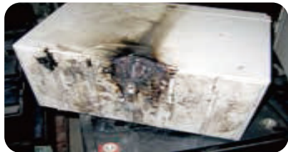
Leakage from battery bottom
