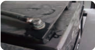
Terminal acid leakage
