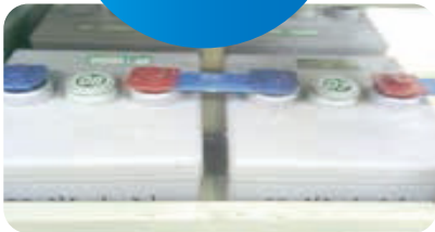
Leakage from battery cover
